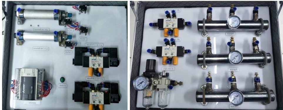
Figure 1: Experimental set of wind pipe separation control with PLC
